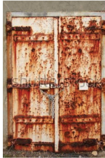
Corroded door (sign of bad engineering design) due to inadequate assessment of environmental conditions or wrong surface treatment
